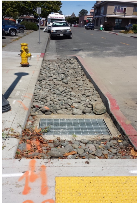
TDA- Stormwater Infiltration Gallery
